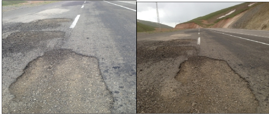
Figure 4. Deformation points on Erzurum-Bingöl road surface.
